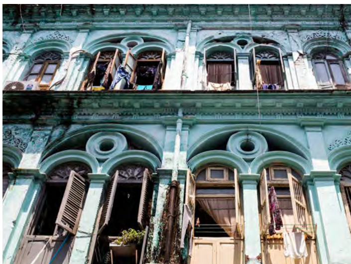
Example of unrestored Yangon heritage building
