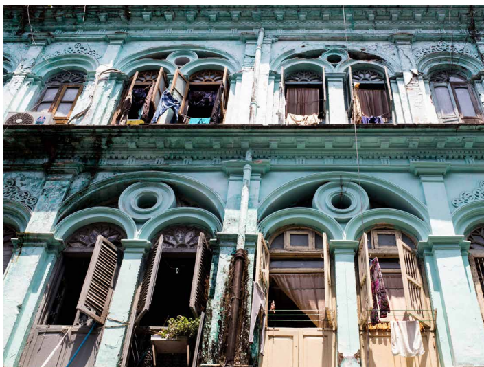
Example of unrestored Yangon heritage building
